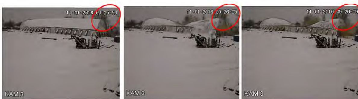
Fig. 2. Progressive collapse of a special-type arch structure
